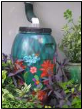
Rain barrel used to collect rain water runoff from a roof.
