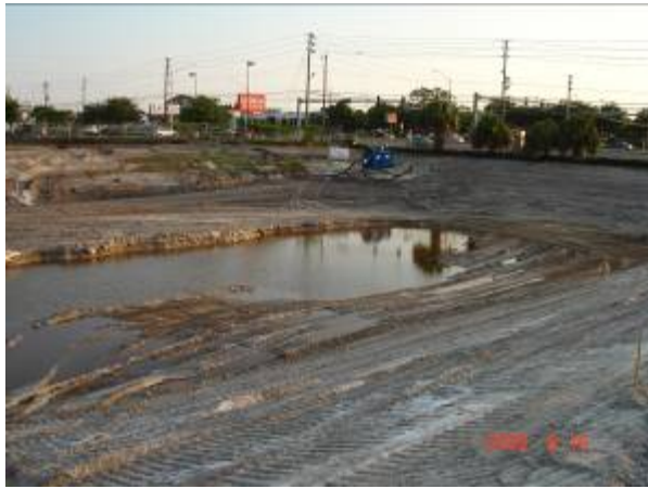
5. Looking southwest towards the adjacent Office Depot during dewatering and excavation process.
