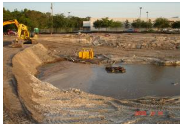
4. Looking south over the middle of the site during the dewatering and excavation processes.
