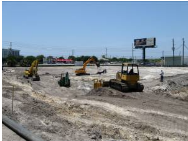
7. Looking northwest from the southwest corner of the site during the dewatering and excavation processes.
