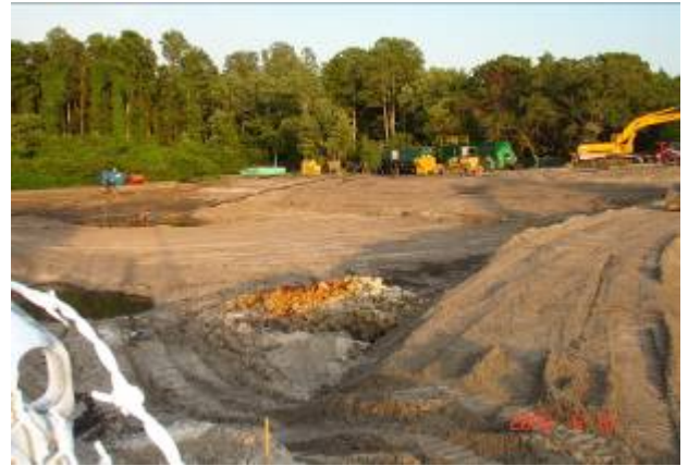
6. Looking east toward the weir. The excavation and dewatering processes are shown in the foreground and background, respectively.
