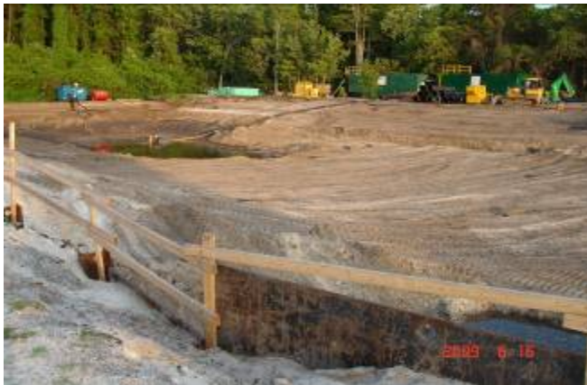
3. Looking southeast toward the outfall weir during the dewatering and excavation processes.
