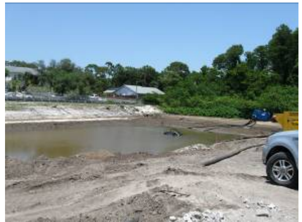
8. Looking northeast from the middle of the site during the dewatering and excavation processes.
