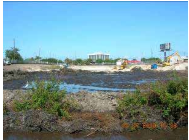
6. Looking west from on top of weir. In the foreground you see the dewatering process and in the background you see the excavation process.
