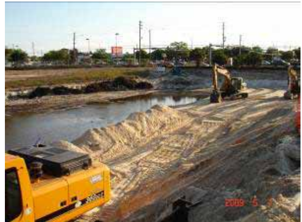
8. Looking southwest from the middle of the site during the dewatering and excavation process.
