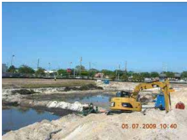
7. Looking southwest from the northeast corner of the site during the dewatering and excavation process.
